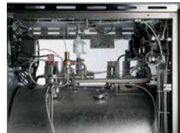
Modulating valve on steam inlet Modulares Ventil am Dampfeinlass
