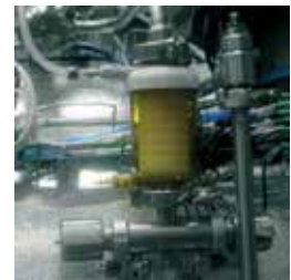
Decontamination of exhaust air with sterile filter / Dekontamination der Abluft über Sterilfilter
