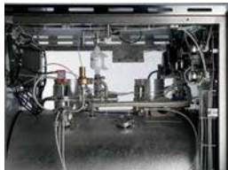
Modulating valve on steam inlet Modulares Ventil am Dampfneinlass
